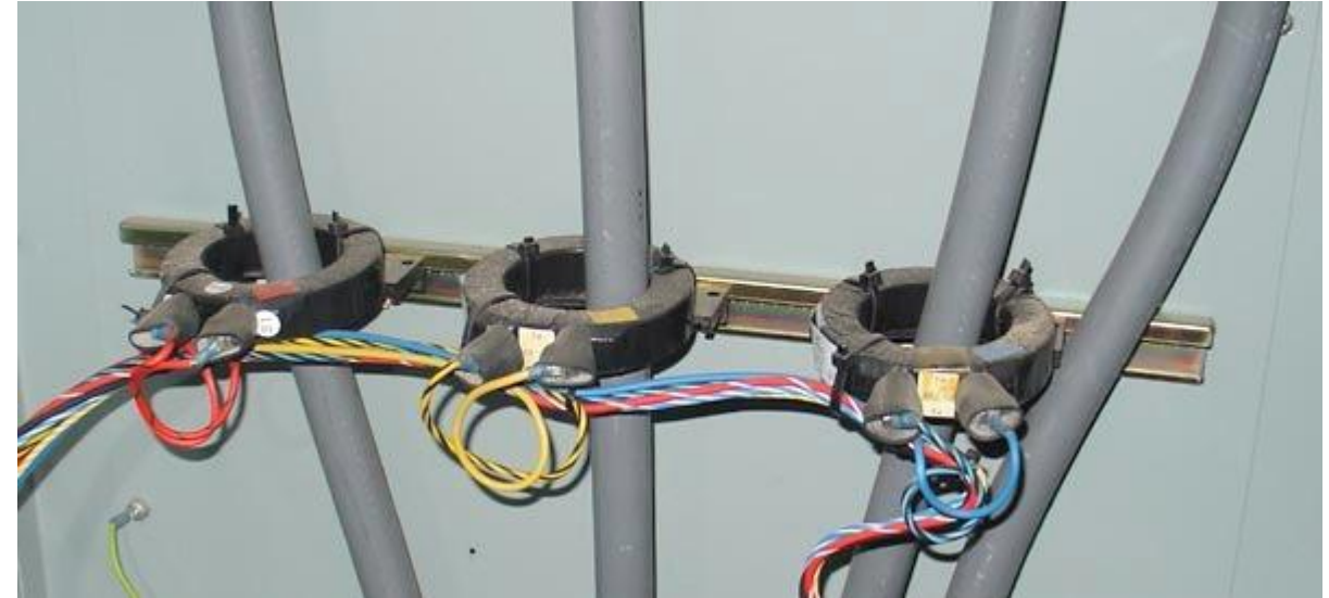
Fig. Current transformers used in metering equipment for three-phase 400-ampere electricity supply
